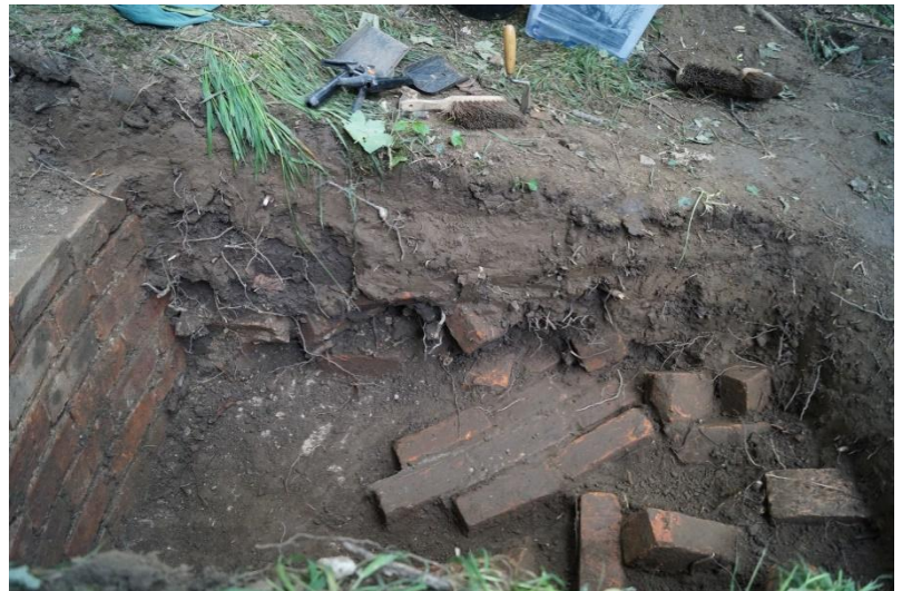
Figure 97. Fallen brickwork revealed in side trench.
