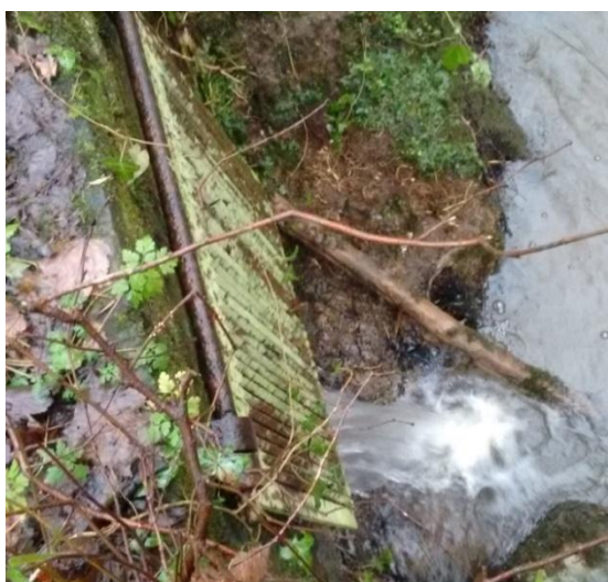
Figure 17. Water flowing out of inlet sluice due to a high level in the pond.
