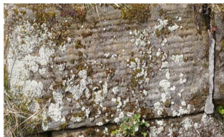
Figure 41. Ashlar corner blocks.
