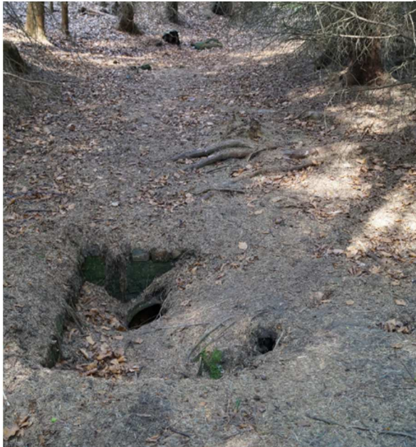
Figure 40. Tullygarth burn manhole.
